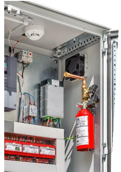
Fig. 12. FFES inside the panel.
