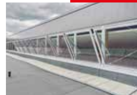
SMOKE EXHAUST WINDOWS
